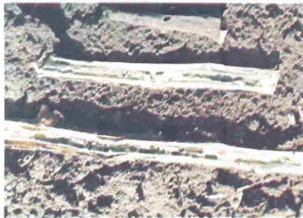
(c) Damage induced by termites
