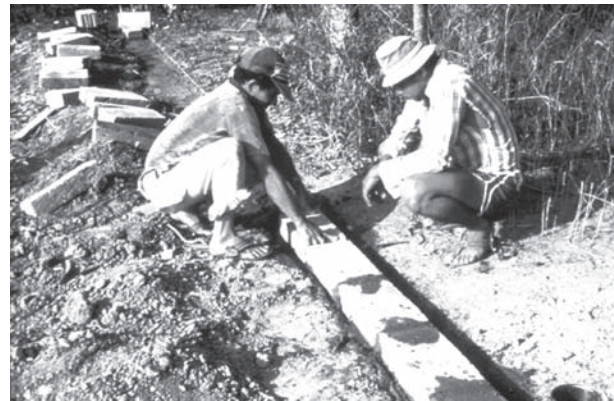
Figure 21-20. Laying down a foundation to support the external walls of a storeroom.
